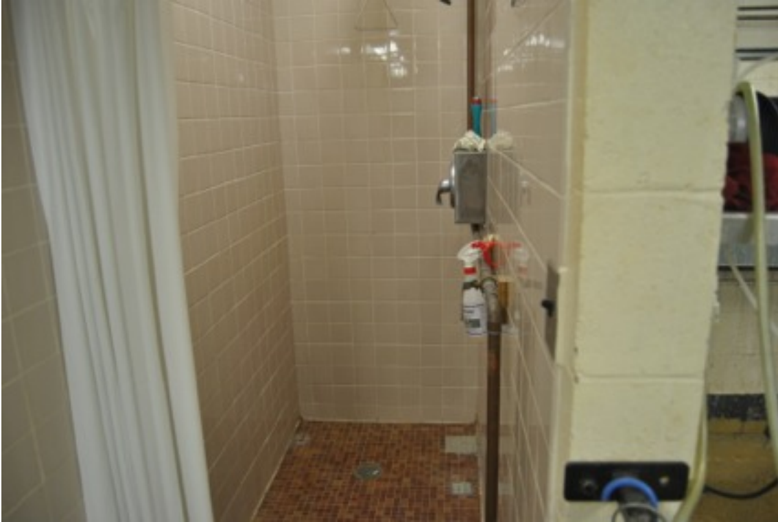
Central Services Level One - Emergency Shower (Potential to be Changed into a AT Shower Facility)
